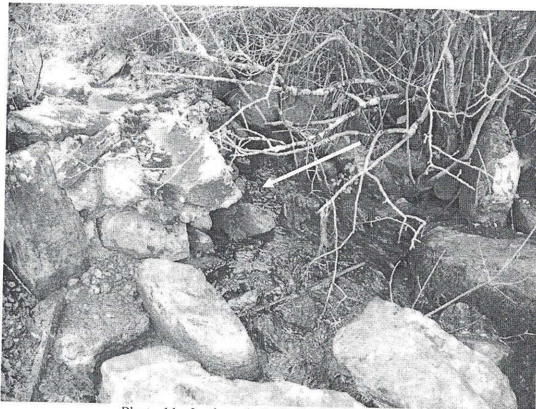
Photo 11. Leakage in Left Abutment (Arrow).
