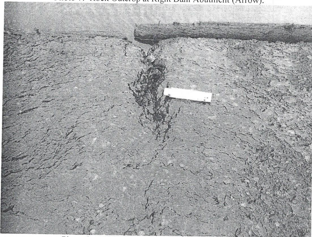
Photo 8. Apron Slab Erosion in Left Spillway Bay.
